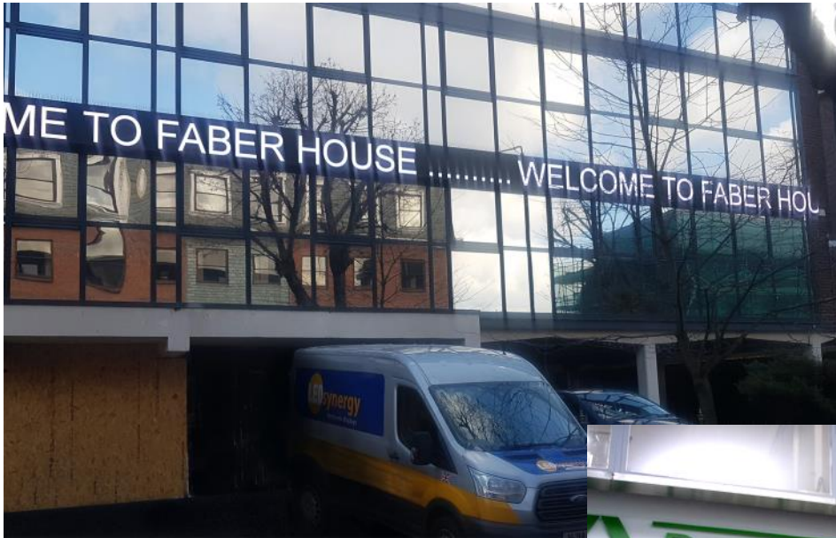
Left: Ticker Display installed to front of building, white LEDs
